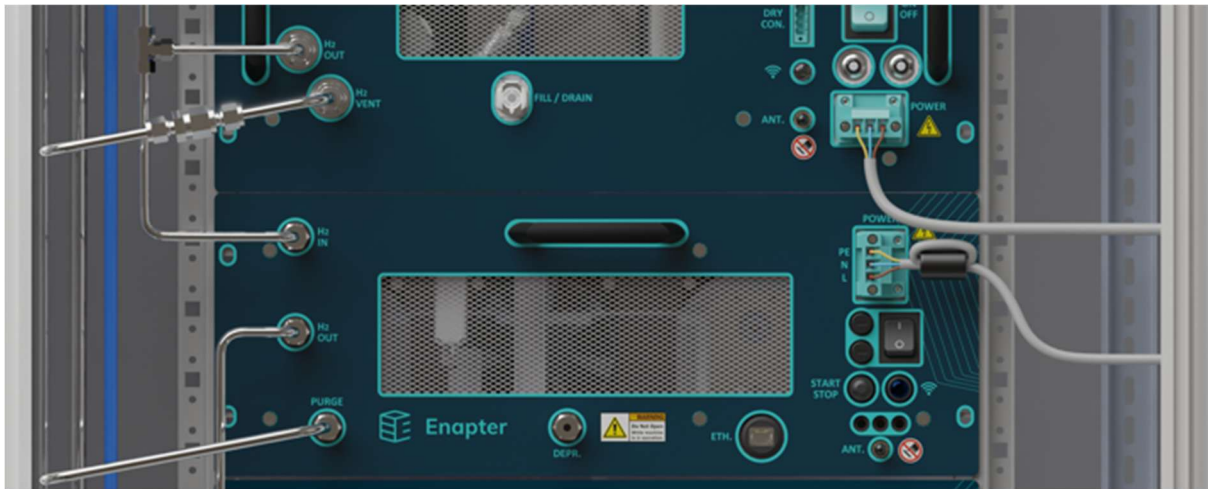
EL and DR Purge line connected
